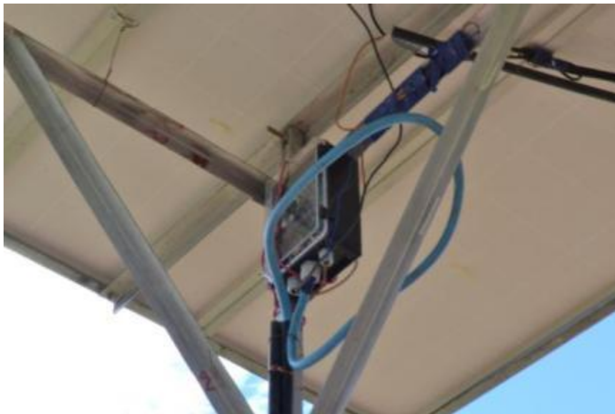
Figure 3: The “brains” of the system are contained within this simple control box that measures and regulates the electricity which runs the pump, monitors water tank levels in two tanks, and protects the pump from running dry.
