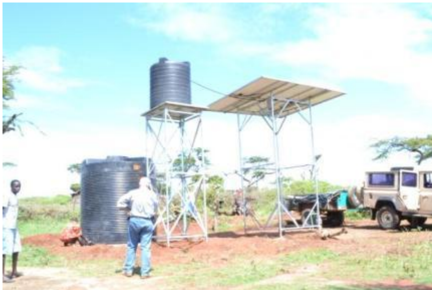
Figure 5: The 1,000L tank feeds the 10,000L tank which also has its own full sensor.
