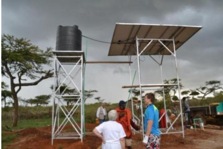
Figure 4: Water is first pumped up to an elevated 1,000L water tank. The controller will sense when the tank is full and stop the pump operation.
